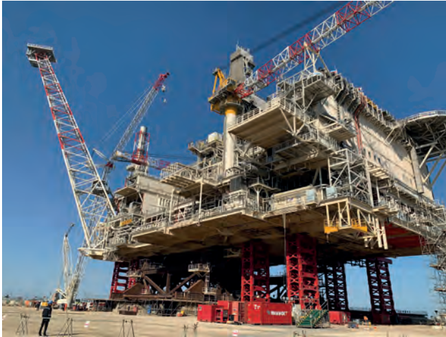
ACE platform topsides jacked up on the load-out frame waiting to be loaded onto transportation barge and sailed away offshore.
